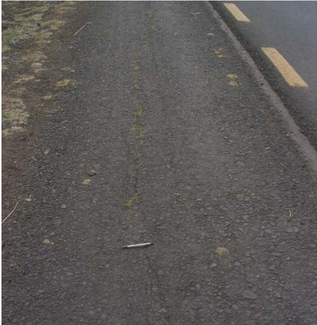
Fig. 1. Longitudinal cracking in the shoulder
