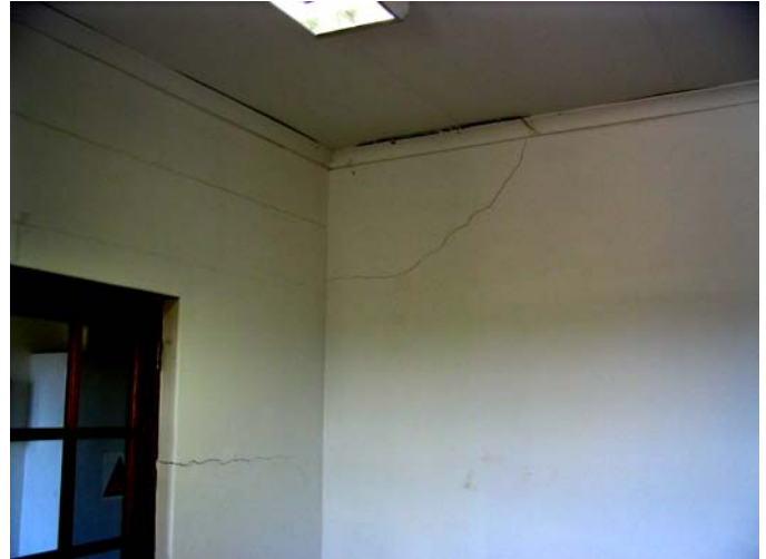
Fig 7. Cracking parallel to ring beam (above window) and on internal wall
