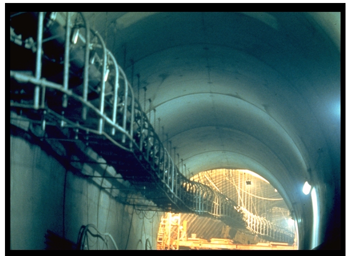
Fig. 6: Underground elevated conveyor belt
