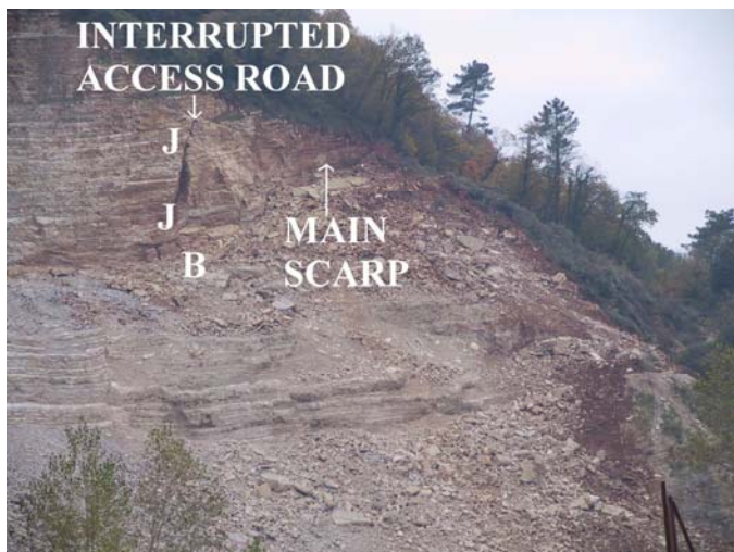
Fig. 3 Picture taken on 22 nd November 2004 of the collapsed zone after the failure: JJ sub-vertical joint, B Block
