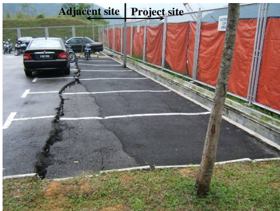
Fig. 22. Site conditions of adjacent lot after the incidence of wall and ground distresses (Northern view).
