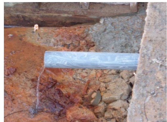
Fig. 9. Continuous seepage flow.
