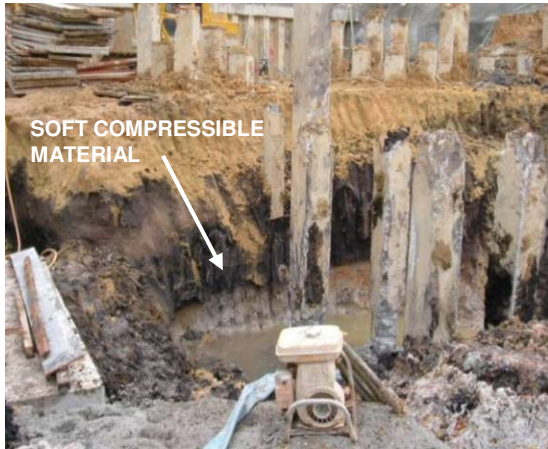
Fig. 10. Soft compressible material detected at localized pile cap excavation.
