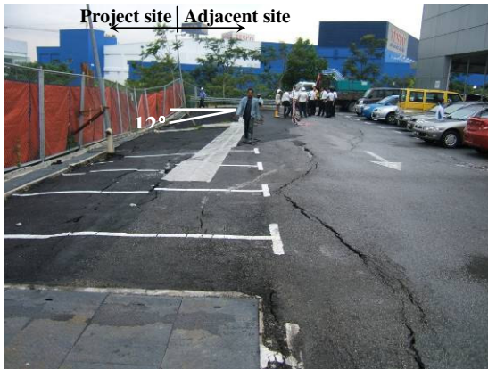
Fig. 21. Site conditions of adjacent lot after the incidence of wall and ground distresses (Southern view).
