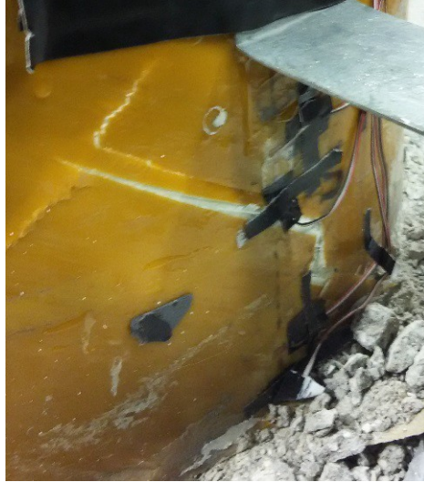
Figure 7 — FRP rupture of the column F4-24-E344-RS at a lateral drift of 14.5%
