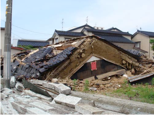
Figure 7. Photograph of house collapse at site NIT-55 that is linked to the thumbnail image in the balloon in Figure 6
