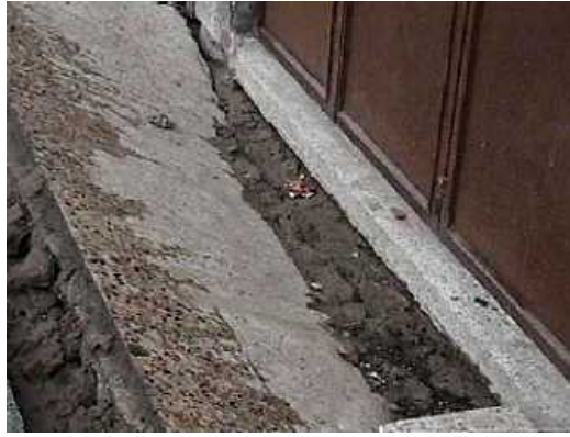
Fig. 1. Sand boils observed at the edges of structures (photos from nieese.berkeley.edu)
