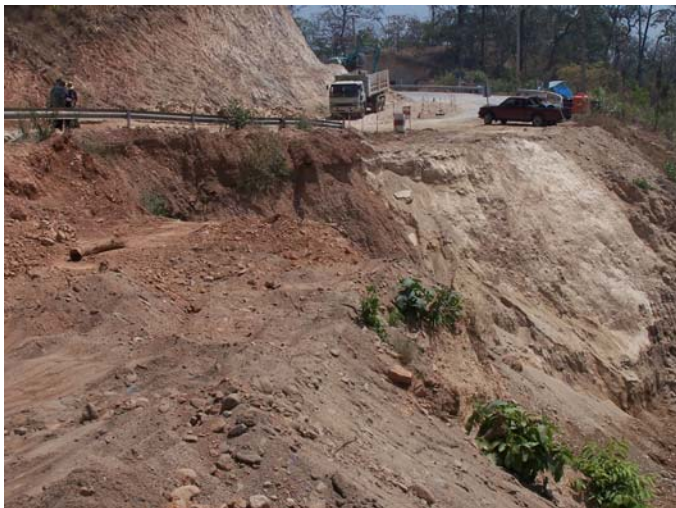
Figure 2: Site with Sloped Embankment Failure
