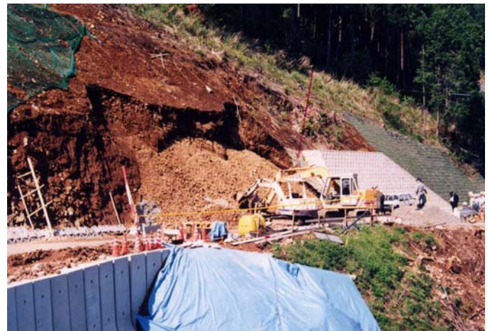
Fig. 1. Labor accident caused by slope failure.
