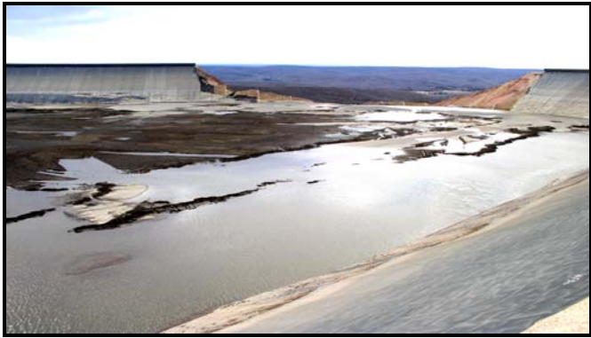
Fig. 3. View of breach looking northwest across reservoir (Hoffman, 2005).
