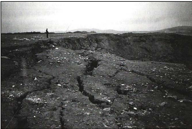
Fig. 4. Tension cracks on top of landfill and steep backscarp in MSW after slope failure (Kocasoy and Curi 1995)
