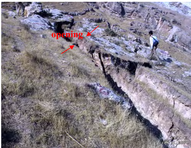
Fig. 9. The appearance of vertical joints in the southern wall of affected area and on the ground surface
