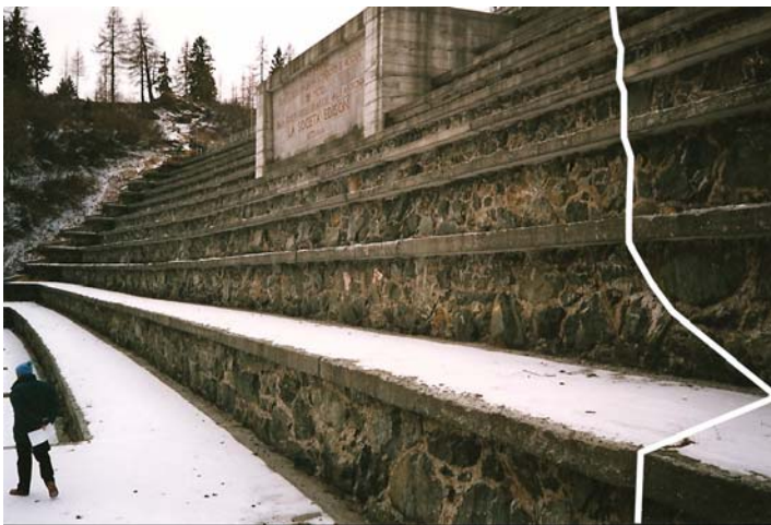
Fig. 4. Down stream abutment of Alpe Cavalli dam with indication of the observed vertical crack.
