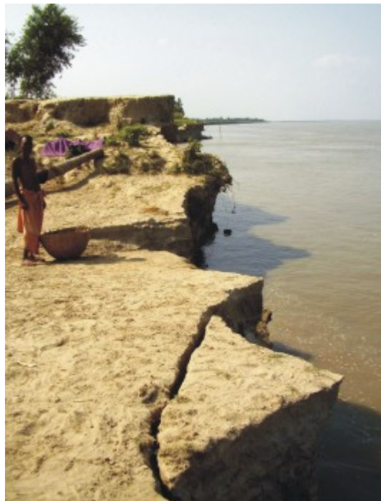
Fig.3. Jamuna flood control embankment in Bogura, The Daily Star 2007/05/02
