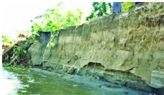
Fig.4. Padma river embankment damages at Rajbari., Naya Digonta 2007/06/16
