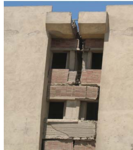
Figure 12. Rupture of beam and column near expansion joint of a reinforced concrete building in Egypt.
