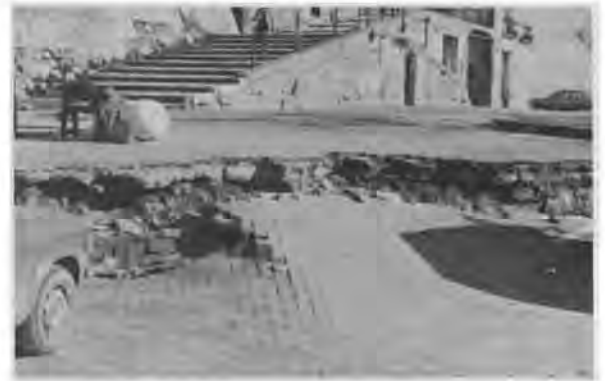
Fig. 7. Permanent vertical displacement at top edge of the landslide in Calitri
