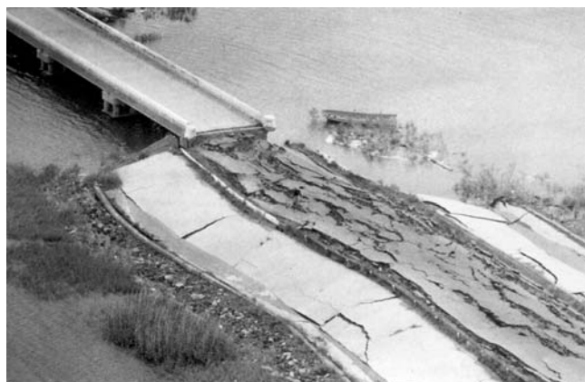
Fig.4. Bridge on undamaged pile foundations with failed approaches due to liquefaction (Finn and Fujita 2002).
