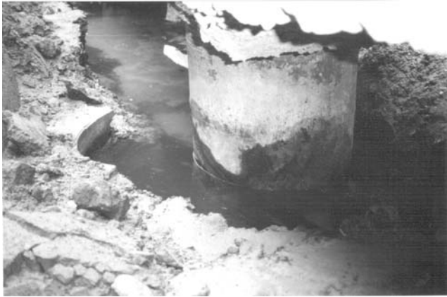
Fig.5. Undamaged pile supporting a crane rail in ground that moved about 1m (Finn and Fujita 2002).
