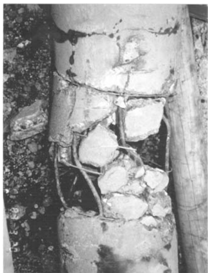
Fig.2. Damage to pile by 2m of lateral ground displacement during 1964 Niigata earthquake (Yoshida et al. 1990).
