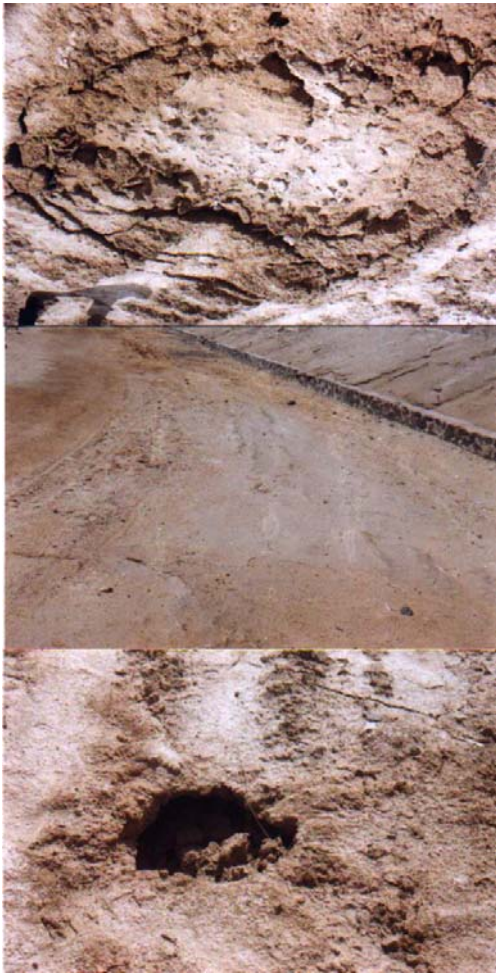
Fig. 7 Location from where the salt and water oozed out at salt factory at Bachau
