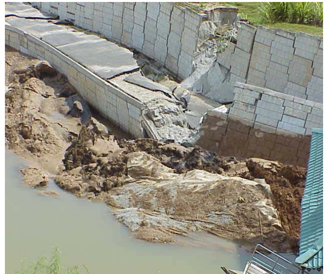
Fig. 4. Collapse of the two RE wall due to the slope failure
