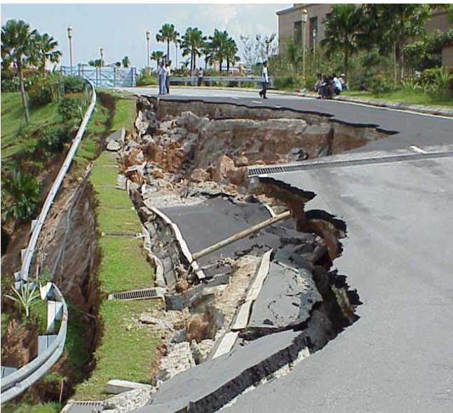
Fig. 3. The top portion of the failed slope
