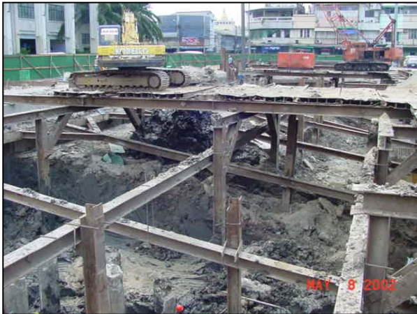
Fig. 16. View of raker and soil-berm support – soil-berm was removed locally in bay
