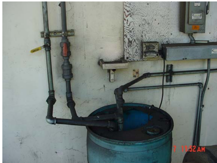
Figure 12 Drum for collecting condensation
