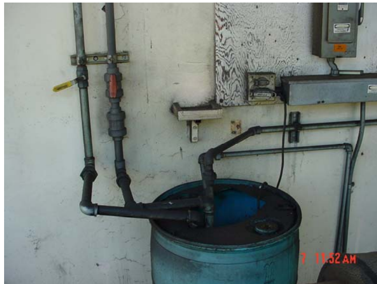
Figure 12 Drum for collecting condensation
