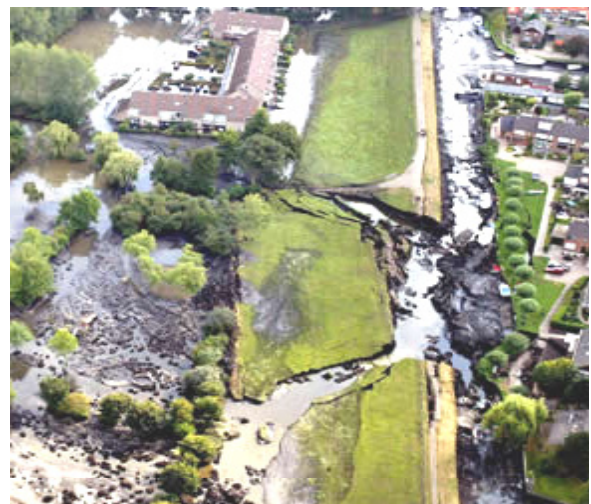
Fig. 2. Shifted part of a canal dike
