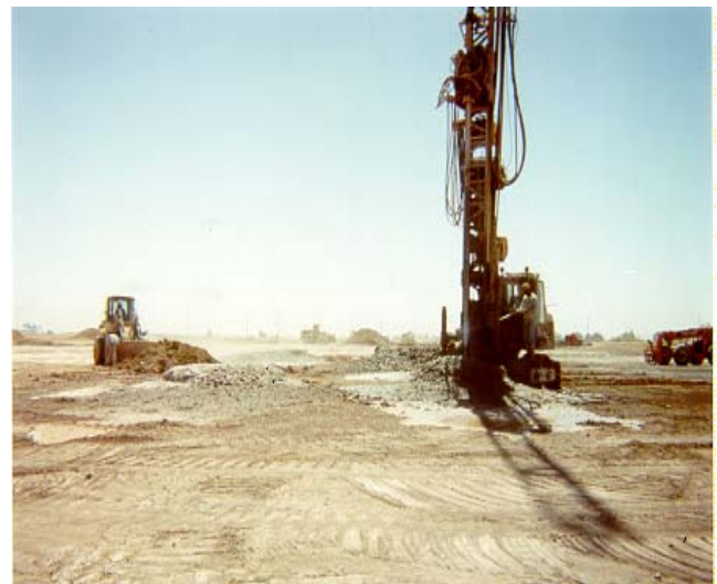
Fig. 4. Spoil Material From Jet-Grouting Being Loaded for Transport to Cooling Tower Foundation Area.
