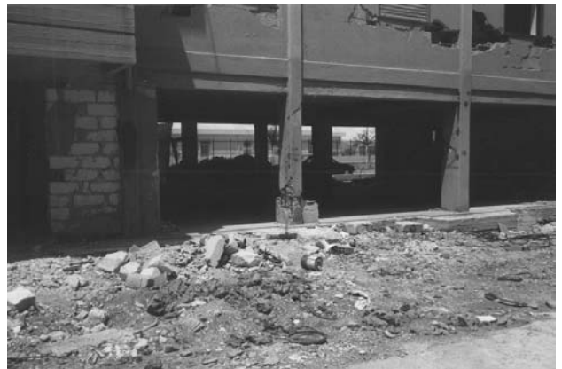
Fig. 2. Damages occurred on buildings.
