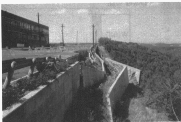
Fig. 2 View of the Failed Section of Wall
