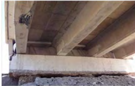
Fig. 4.7 Damage in Chada Bridge with no diaphragm.
