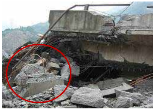
Figure 67. Photo. Column Shear and Flexural Failure at Bent 15.
