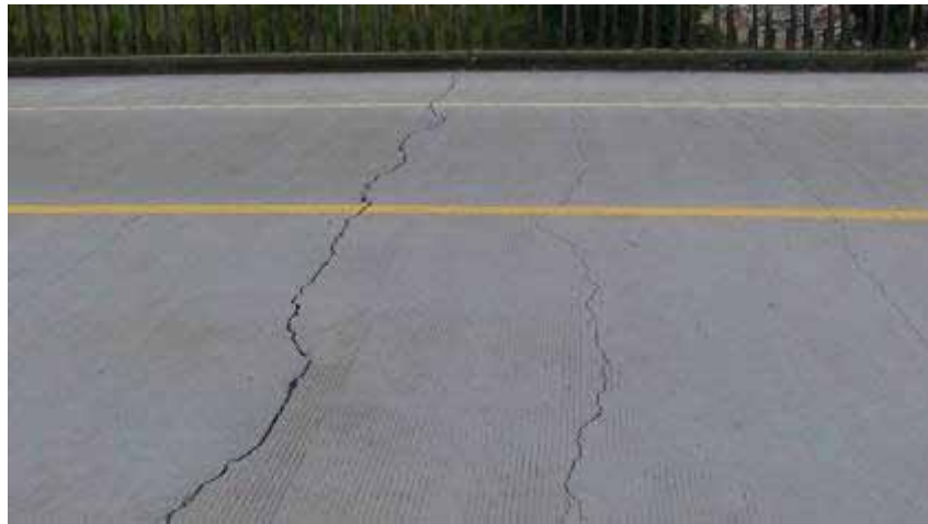
Figure 23. Photo. Transverse Crack on Top of the Bridge Deck in Span 3.
