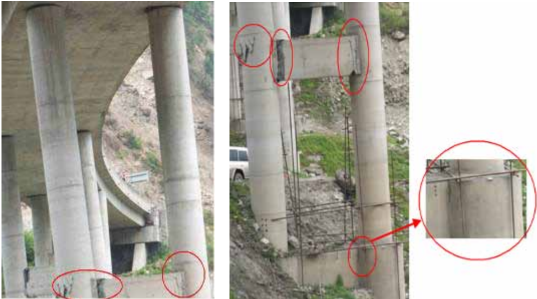
Figure 65. Photo. Damage at Bent 3.
