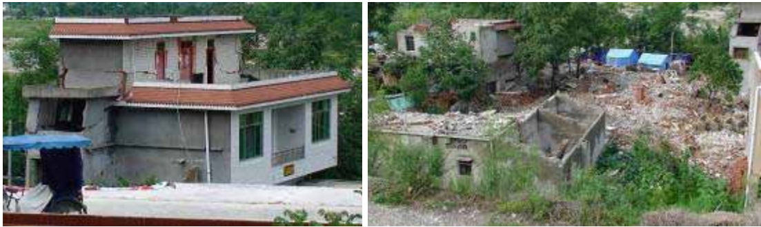
Figure 33. Photo. Building Damage in Nearby Town.
