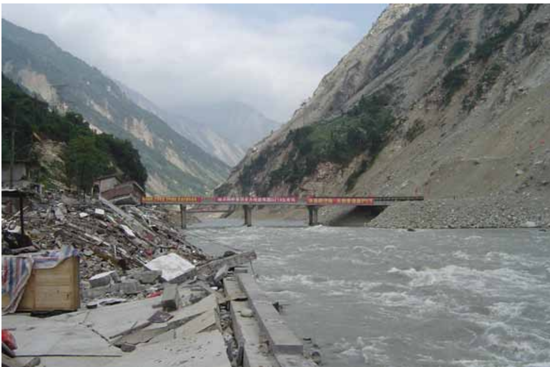
Figure 62. Photo. Mingjiang Bridge and Other Structural Damage in Yingxiu Village.
