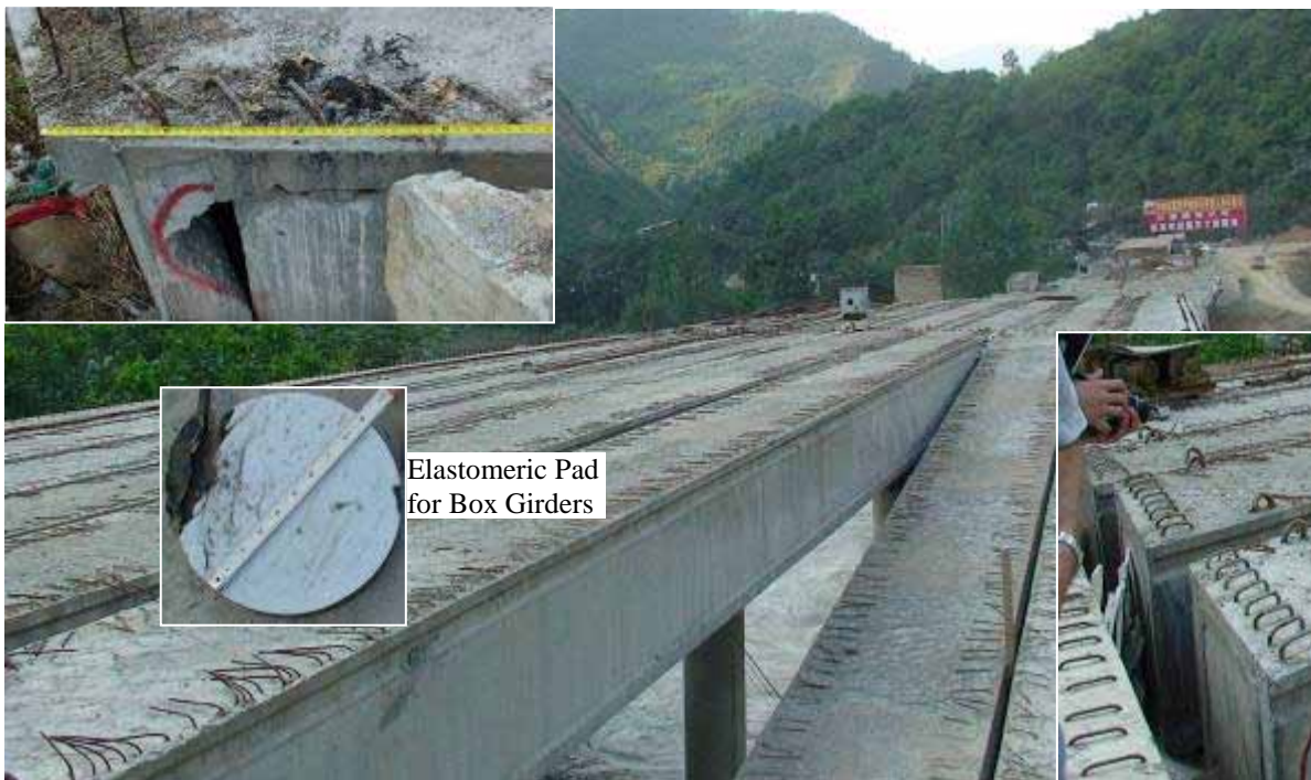
Figure 48. Photo. Damage to the 10-Span Bridge Under Construction.
