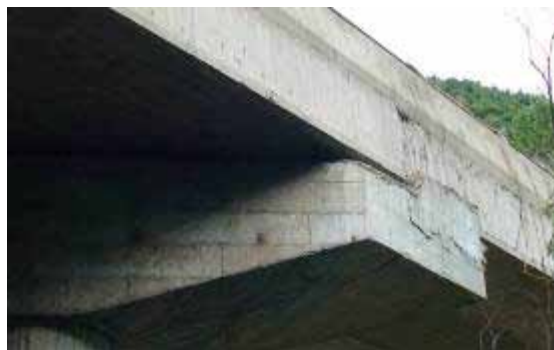
Figure 31. Photo. Damage in Shear Key.
