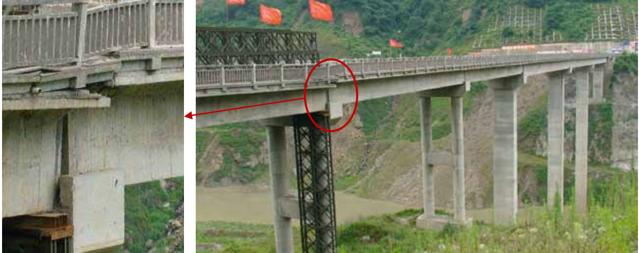
Figure 75. Photo. Overview of the Bridge Structure and Damage Location.
