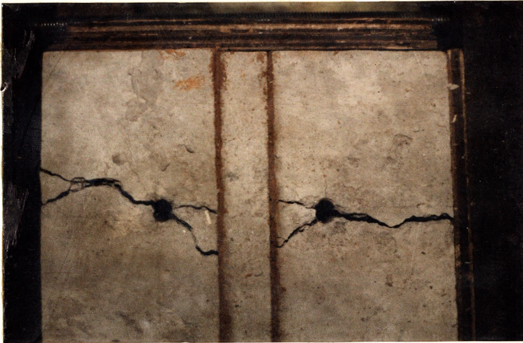
Figure D-13: 1/16 in. Clay Filled, Two-Joint Concrete Model Test: Test C-29, S=4 in., A Failure
