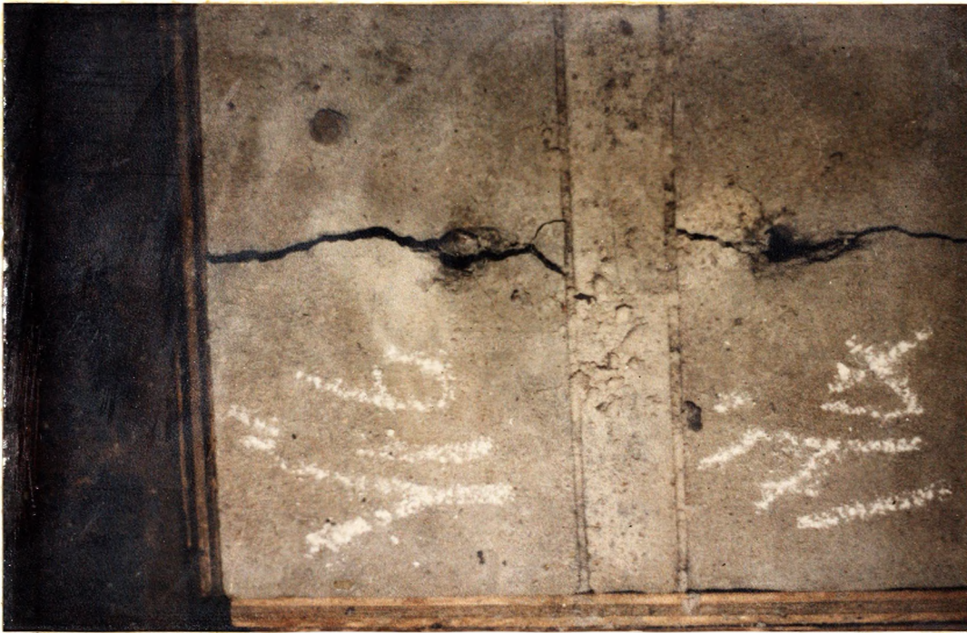
Figure D-7: 1/16 in. Sand Filled, Two-Joint Concrete Model test: Test C-15, S=4 in., A Failure
