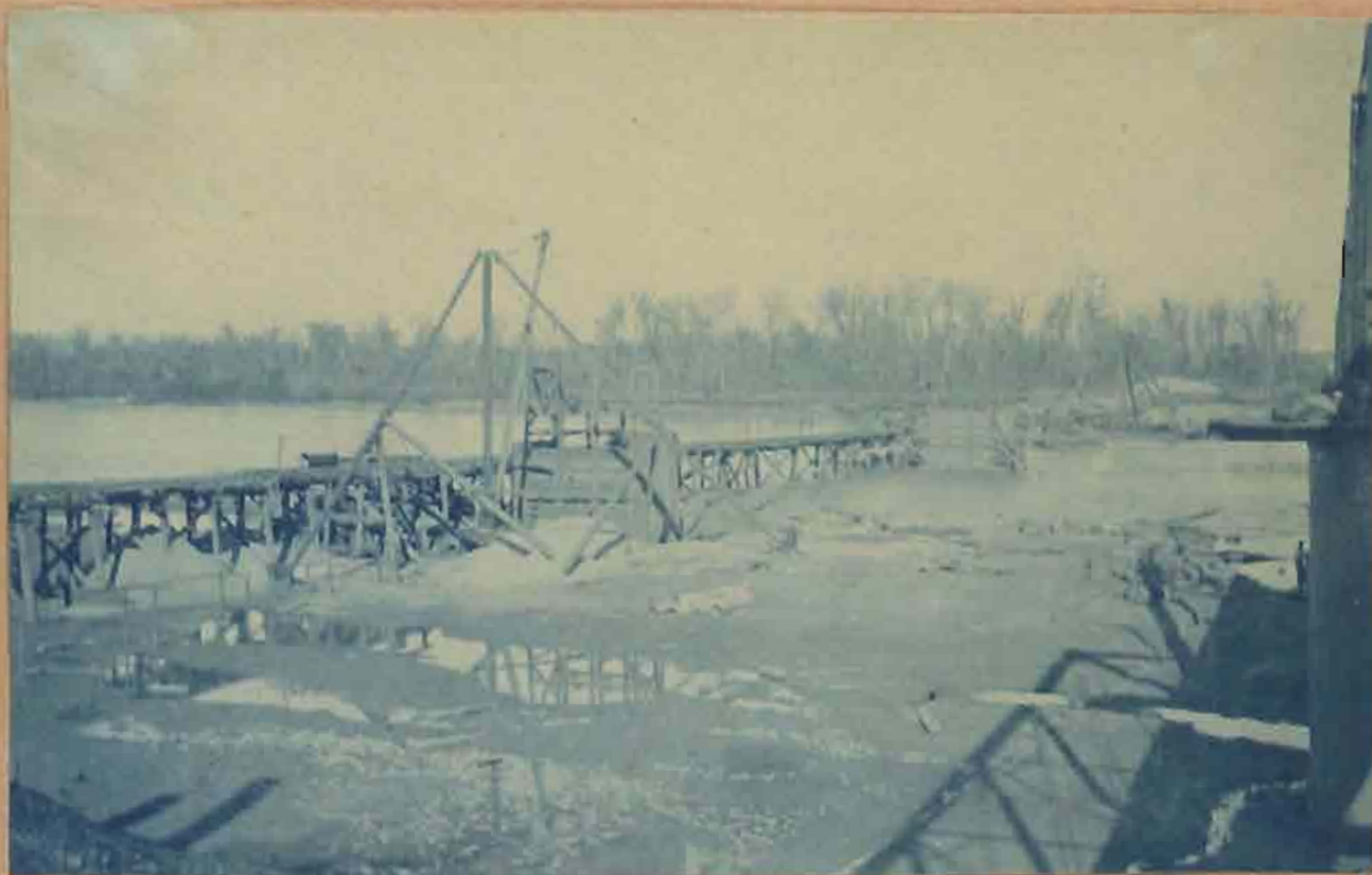
This view shows river just before the second rise 11/16/'99. The forms for piers 6 and 5 respectively are shown in the distance.
