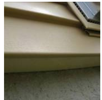
Image2.5: Capped foam edge at the bottom of a wall with metal flashing
