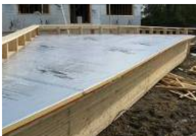
Image 2.6: Rigid foam applied to gable end on the ground than lifted into place with a crane
