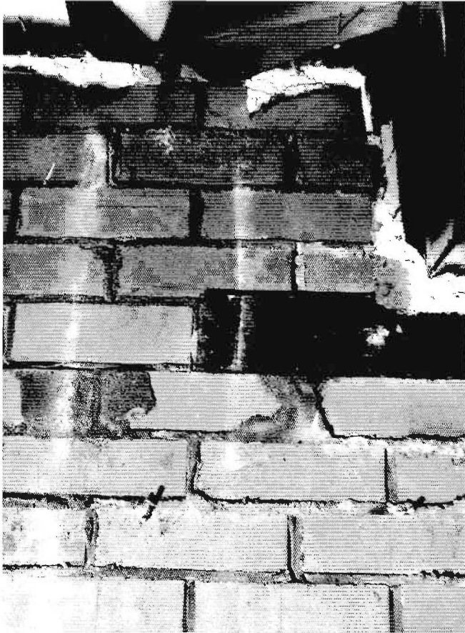
a) Loose Lintel Built Into Veneer Wall
