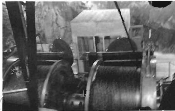
Main Hoist Looking down Cable Raise
