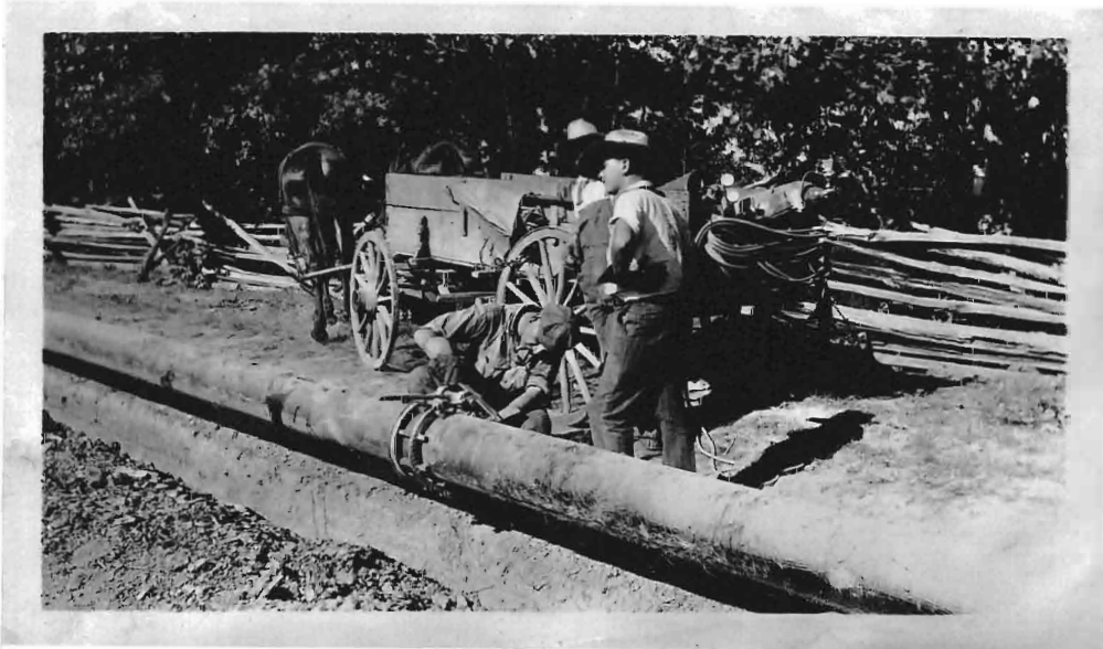
Tacking a Joint Preparatory to Making an Overhead Weld. Note Welding Clamp Holding Pipe in Position
