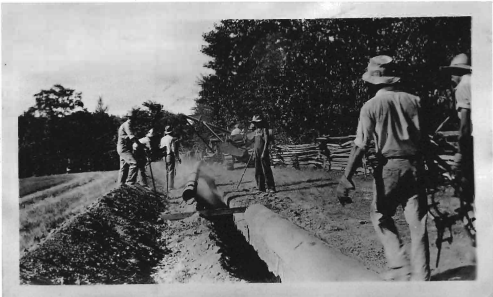
Snaking Pipe Onto Skids Over the Trench With a Caterpillar Tractor Equipped with a Boom.
