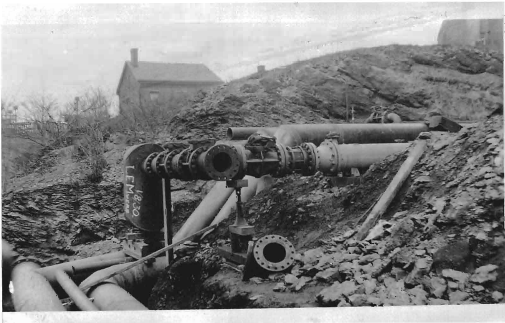
Main Line from Compressors Tying in to After Cooler and 24" Line to Gas Holder
