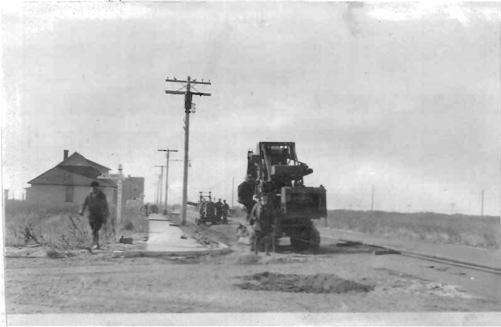
Excavating with Machinery Along a County Road in Southern New Jersey. The Machine in the Foreground is a Barber-Greene With the Bucket Line Set to Remove Six Inches of Top Gravel. Following is a Cleveland Cutting the Trench to a Depth of Thirty Inches
