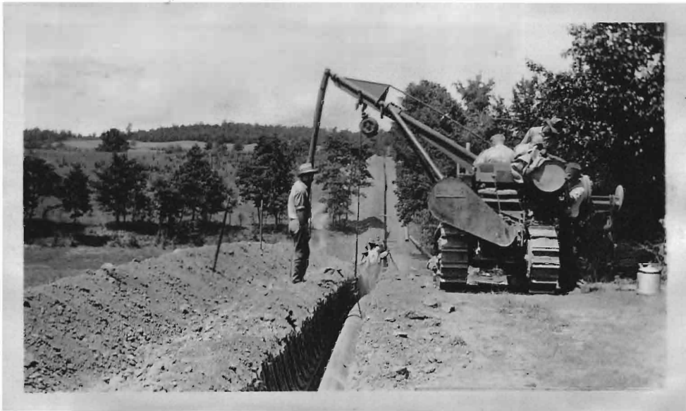
Making an Overhead Bend in a 12" Gas Line With a Tractor and Boom.
