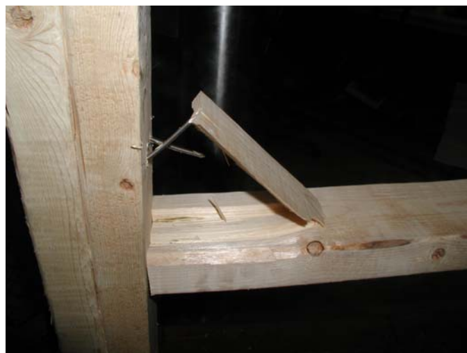
Figure 6 – Failure of Wood Plate at Stud
