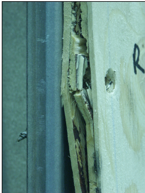
Figure 2.16: Partial Pull Through in Sheathing in Test Wall 40A
