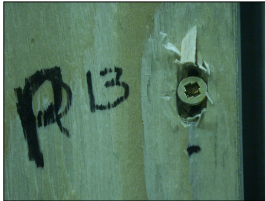
Figure 2.14: Enlargement of Screw Holes in Sheathing on Test Wall 38A
