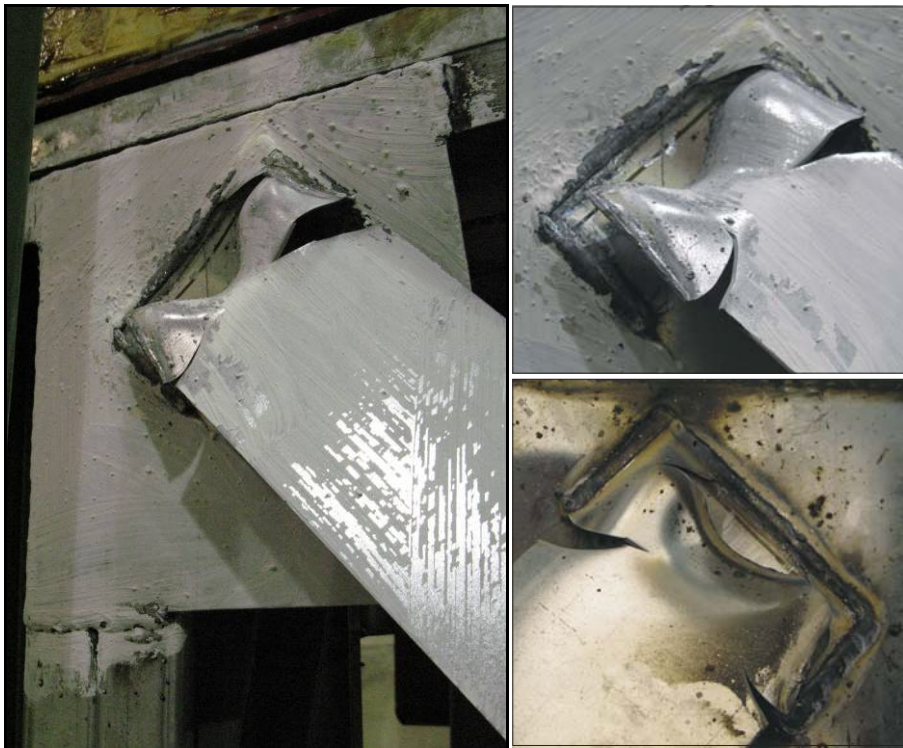
Figure 2.13: Connection failure of preliminary test 21A-M
