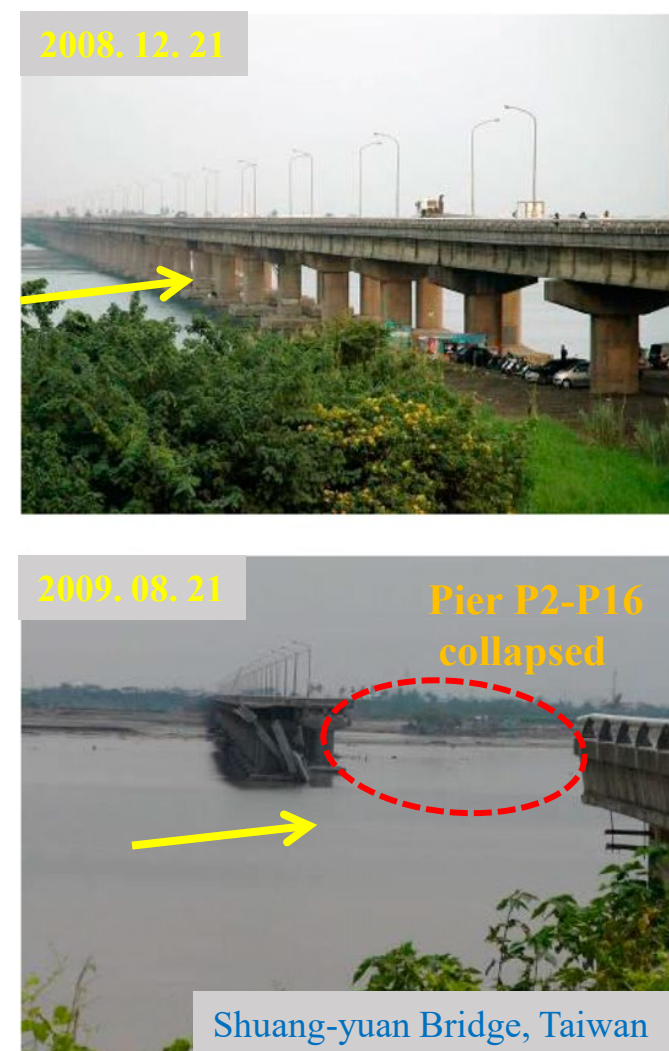
Typical bridge scour accident
