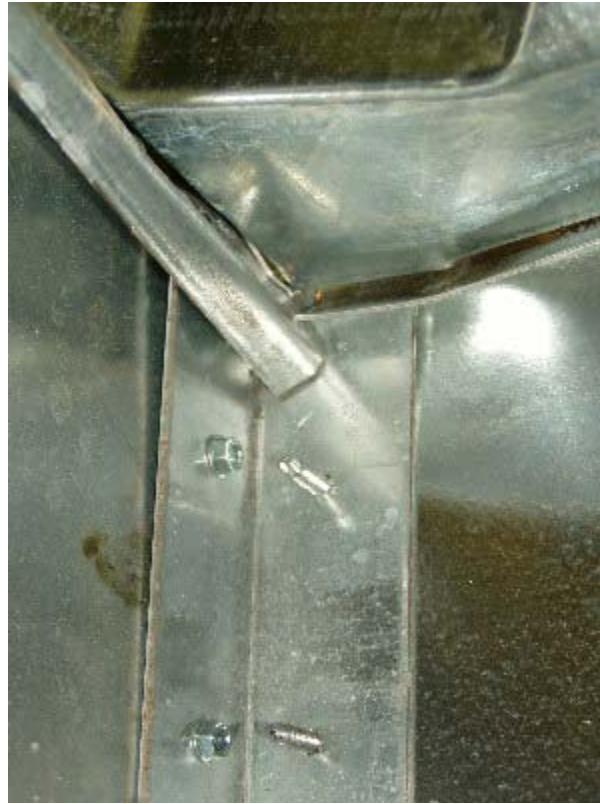
Figure 5.4: Photograph of Track Shear Failure
