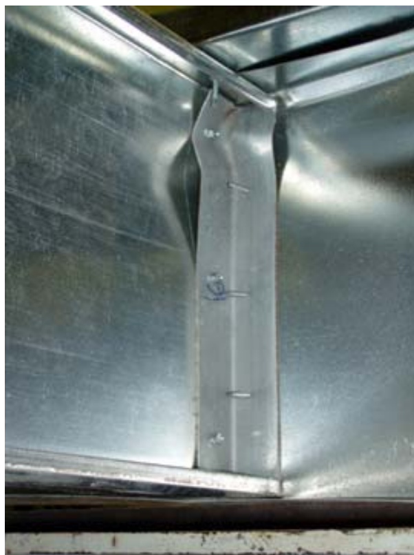
Figure 5.1: Photograph of a Clip Angle Failure
