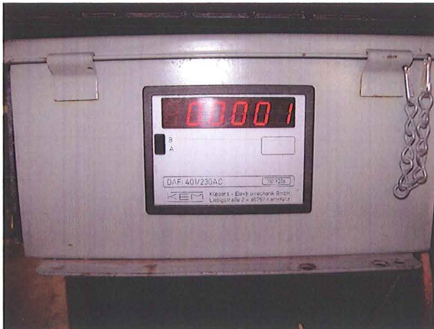
Figure 3.11. Display unit for flow through turbine flowmeter
