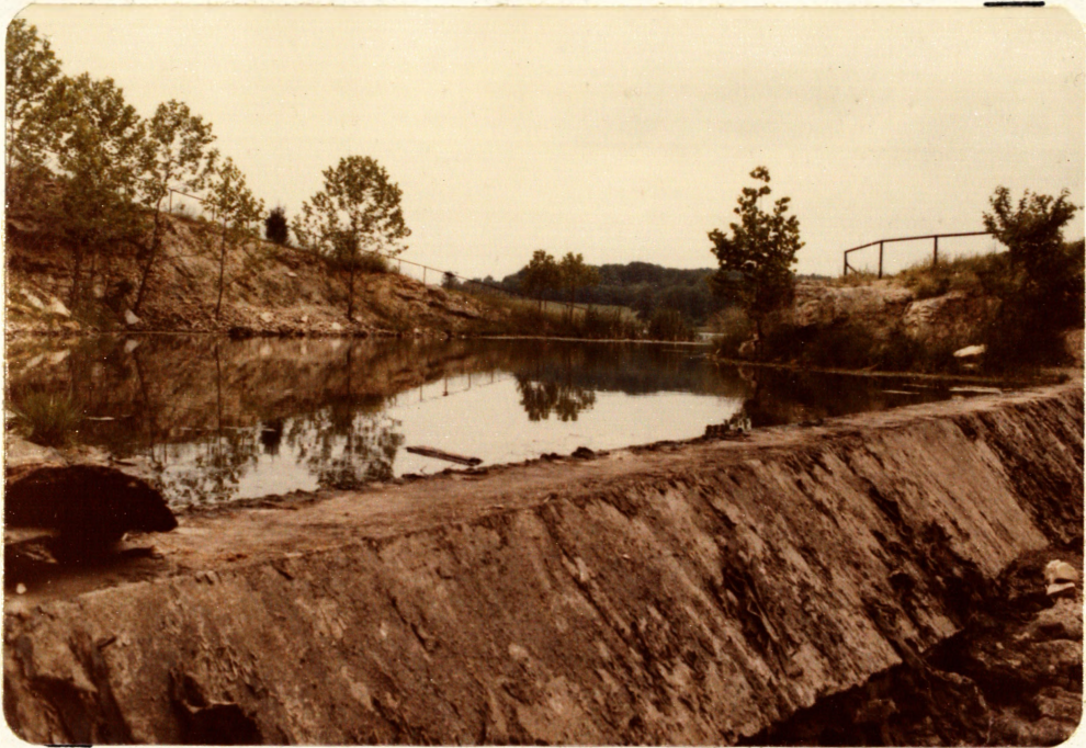
PHOTO NO. 10 - UPSTREAM FROM RIGHT END SHOWING CONCRETE SILL IN PRINCIPAL SPILLWAY
