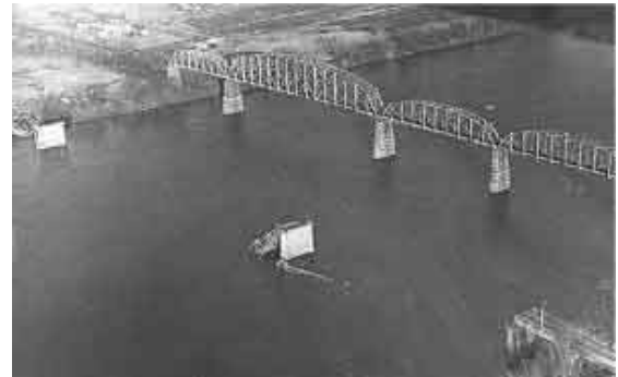
The 1460-foot Suspended Portion Collapsed into the River [4]
