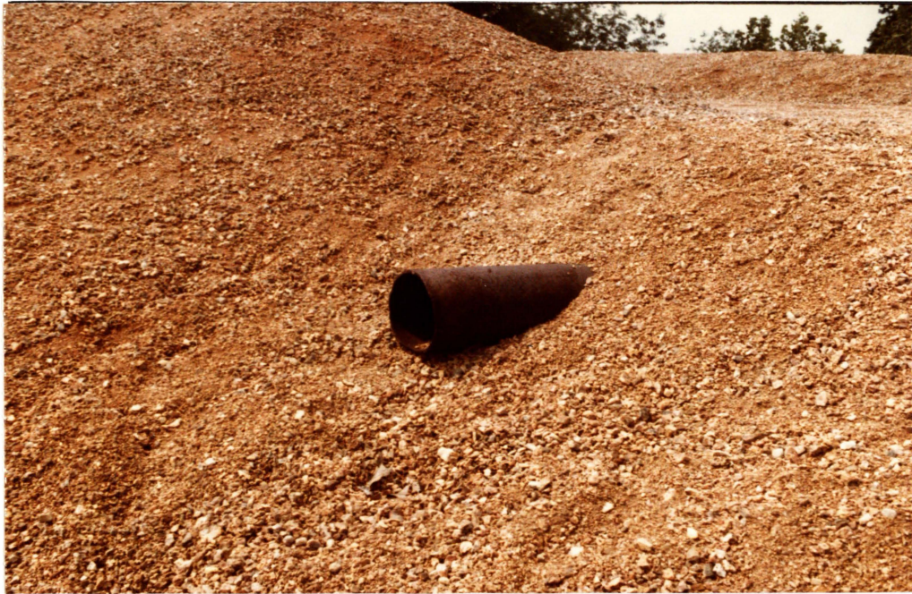
5. Inoperative outlet pipe near south end of embankment. Looking south.
