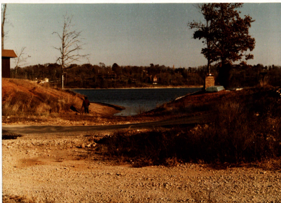
8. Spillway located at right (north) abutment. Note asphalt road across spillway. Looking east from head of discharge channel.
