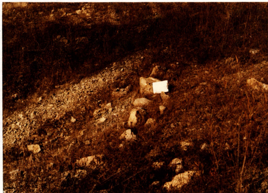
2. Downstream face of dam showing minor rill erosion and material used in construction of dam. Note also variation in density of vegetation cover. Clipboard for scale.
