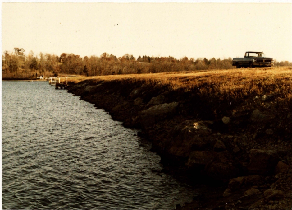
3. Riprap shore protection on upstream slope of dam. Looking southeast from right abutment.
