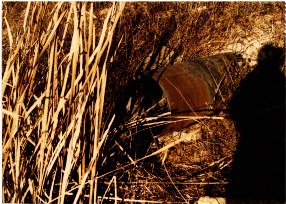
10. 18-inch outlet pipe for outlet structure at left abutment. Pipe flow estimated at 20 gal/min. Looking north.
