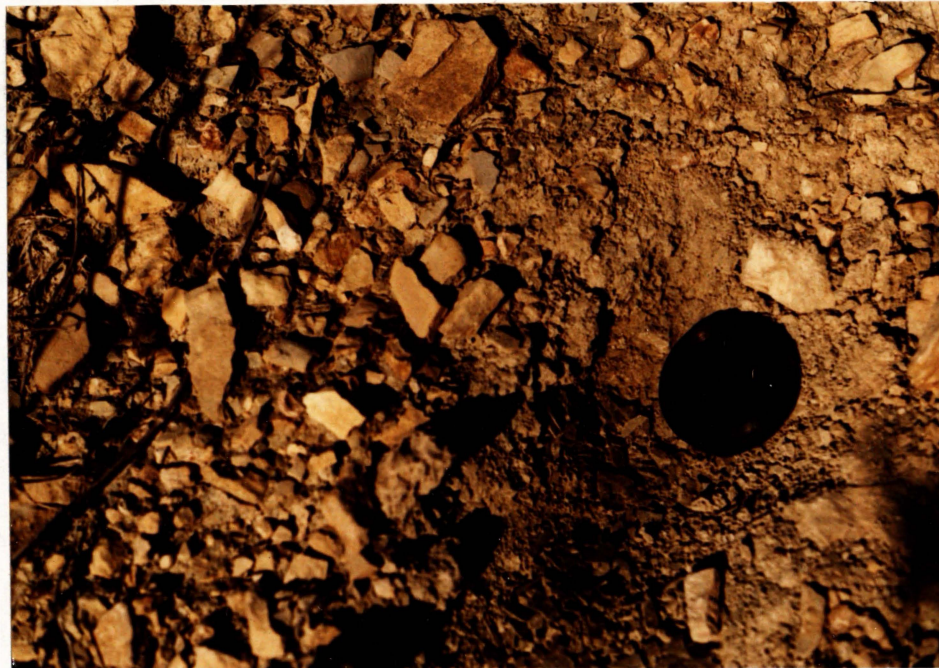
1. Stoney soil used in dam construction. View of downstream face. Lens cover for scale.
