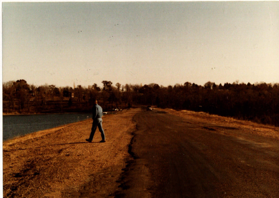
7. Asphalt road on crest of dam. Note broad dam width and lack of any disruption of vertical or horizontal alignment. Looking southeast.
