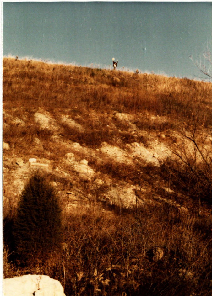
6. Downstream slope of dam showing scattered bare areas and minor rill erosion. Looking northeast from toe of dam.
