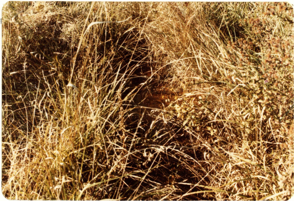
PHOTO NO. 15 - SEEPY AREA AT BASE OF RIGHT ABUTMENT TROUGH
