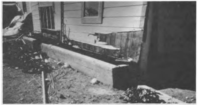
Fig. 2 Damage to House Not Bolted to Foundation
