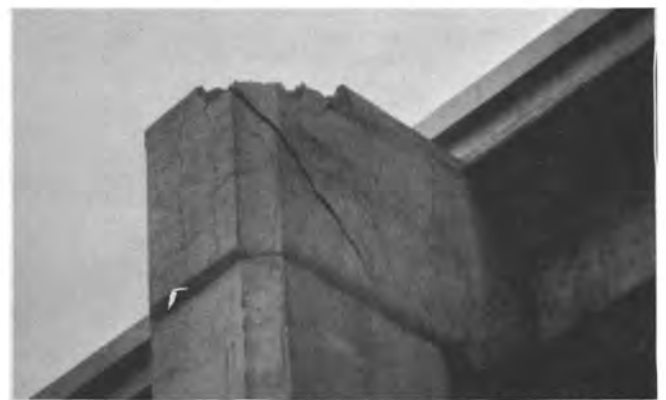
Fig. 25 Damaged Knee Joint in New Freeway
