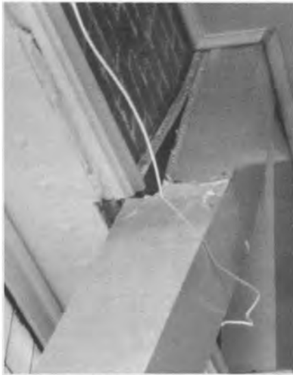
Fig. 16 Buckled Brace in URM Building
