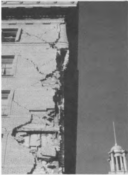
Fig. 14 Damage to Retrofit Steel Frame Building with Masonry Infilled Walls
