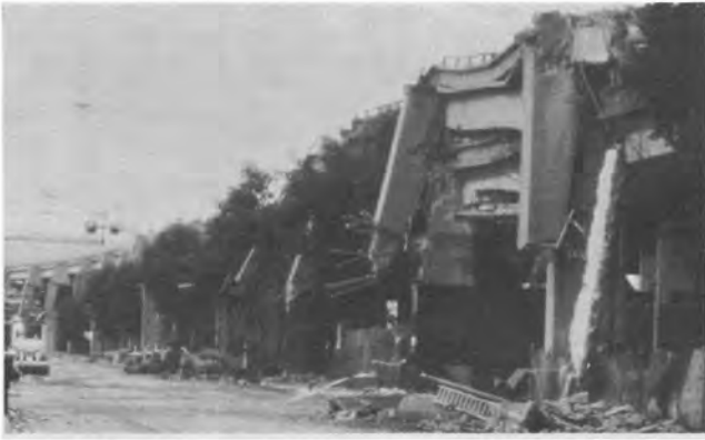
Fig. 20 Collapse of Cypress Street Viaduct
