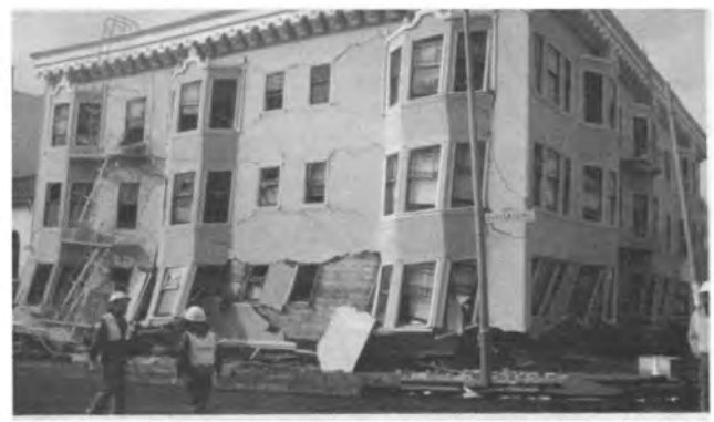
Fig. 5 Collapse of Apartment in Marina District
