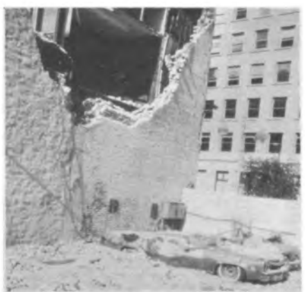
Fig. 7 Out-of-Plane Failure of Masonry Wall
