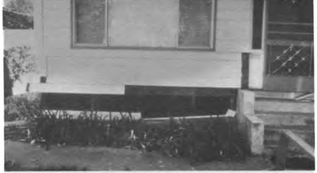
Fig. 3 Damage to "Pony" Wall
