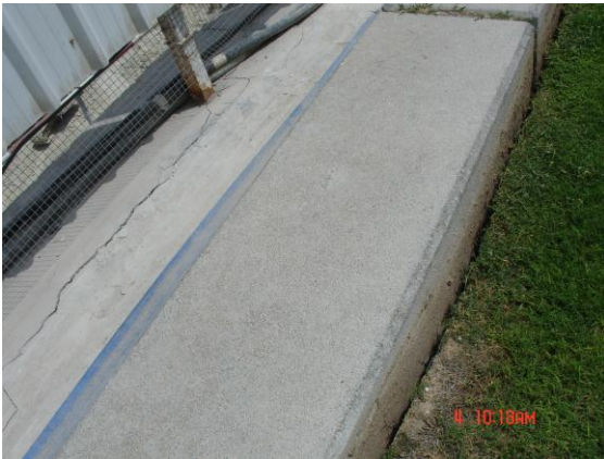
Plate 2. Ground Depression behind Secant Pile Wall
