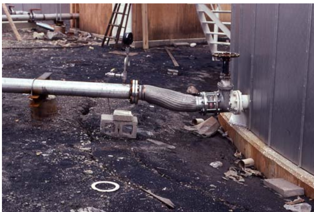
Fig. 8. Flexible connection indicates movement and ground failure
