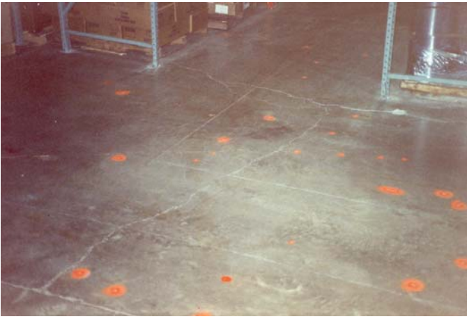
Fig. 4. Warehouse slab exhibiting transverse cracking and popouts (painted orange for identification purposes).
