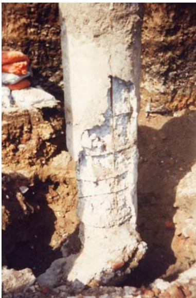
Site 2 Bund Garden, Pune Diesel spillage site
