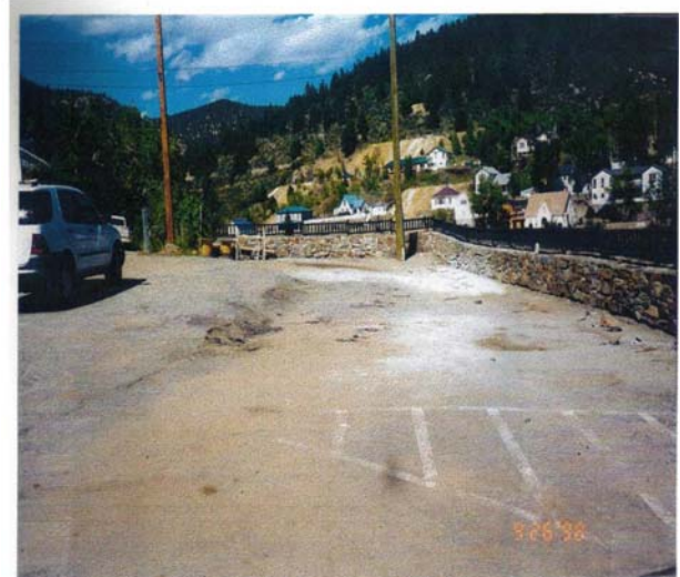
Fig. 1. Settlement at the Wall Crest before Demolition
