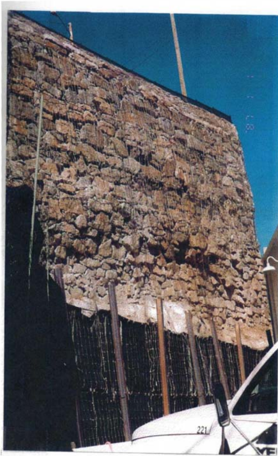
Fig. 2. Lateral Bulging at the Rock Facing before Demolition
