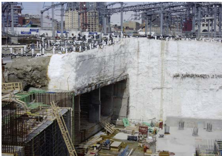
Fig.10 Overall view of the frozen ground support walls and the completed base slab of the cut and cover tunnels.
